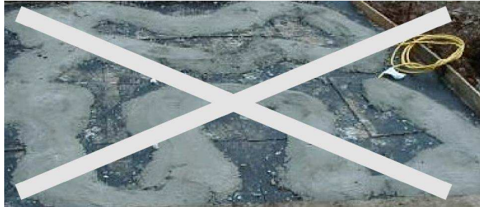
DO NOT cover the cables and the sensors with concrete while waiting for the definitive coverage
