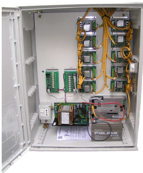
SCA PU + SCA CONTROLLER in the control panel
