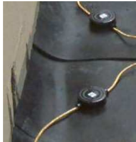
WRONG LAYING - Membrane bent on the wall
