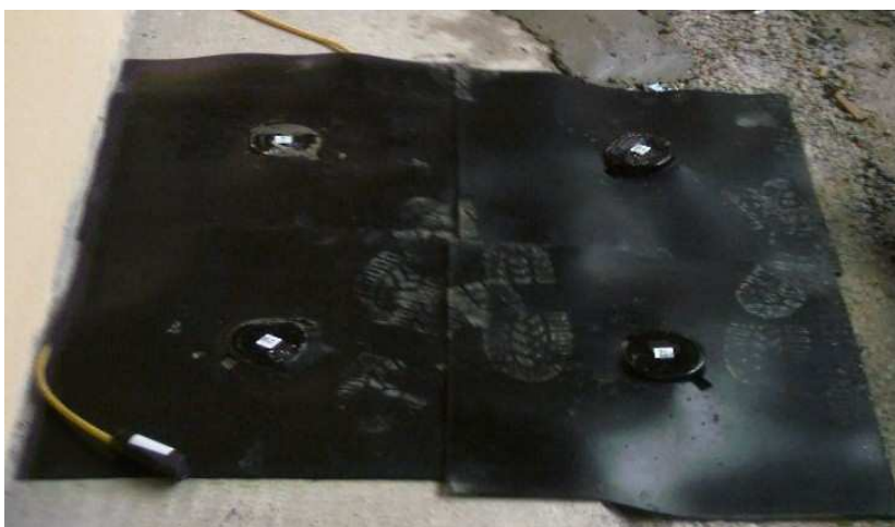
WRONG LAYING – Membranes set after the sensor laying, piled up and on the step
